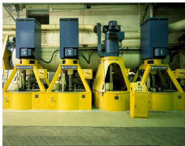
Turbines. Phot. Patrick Glotain IVR22_19936001808VA
