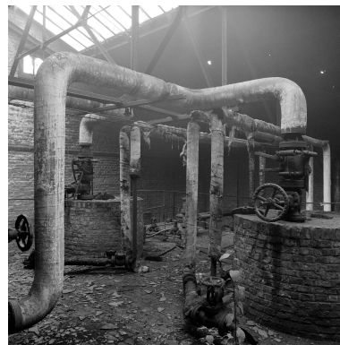
Chaudière, vannes. Phot. Olivier Marlard IVR31_19885902283X
